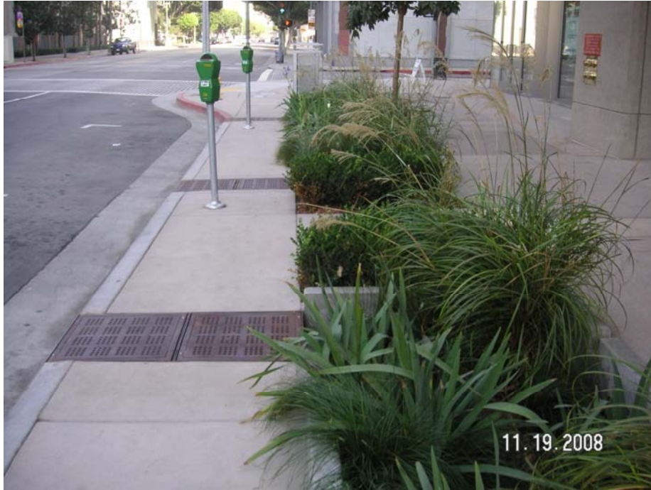
(Curb inlet and infiltration basin in Downtown LA--Hope Street and 11 th Street)
